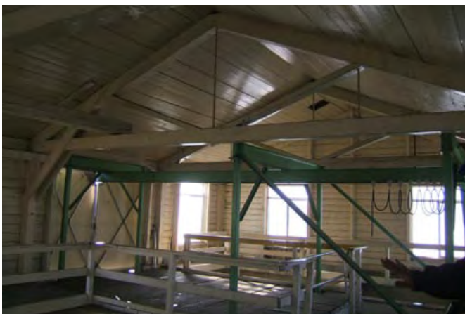
Upper level interior of the Hawley Power House at Willamette Falls during 2005 tour to weigh in on its fate. Unfortunately, the old power house is slated for decommissioning this year by PGE under a FERC order.
