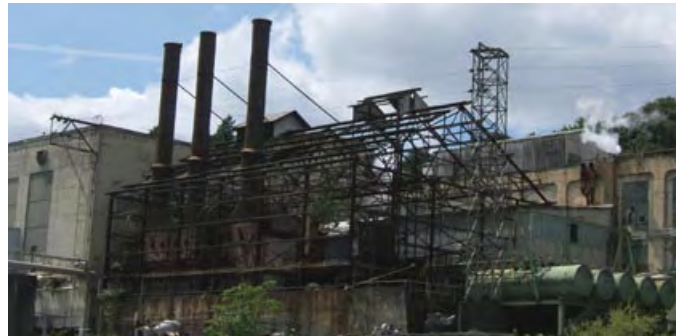
UO architecture students were grateful for their January tour of the West Linn Paper Company's island mill, where they admired the handsome skeletal remains of this old steam plant.
