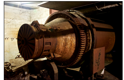
One end of the rotating sulfur burner.
