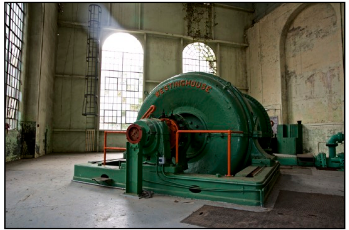
(above) One of the generating units on the main floor of the Bull Run Powerhouse.
