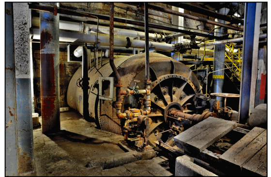
(above) One of the eight water-powered turbines in Grinder Room 2.
