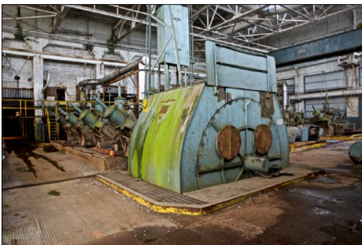
(above) The motor/generator end of one of the grinder lines in Grinder Room #3. These large motors powered the grinders during low water periods and produced power during high water.
