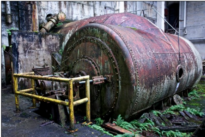
A 10' diameter riveted penstock delivered water to this turbine that originally powered a grinder but was later converted to run one of the dynamos in the Generator Room Annex.
