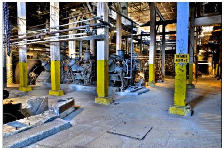
Main floor of Grinder Room #2 showing a turbine to the left and three pocket grinders to the right.
