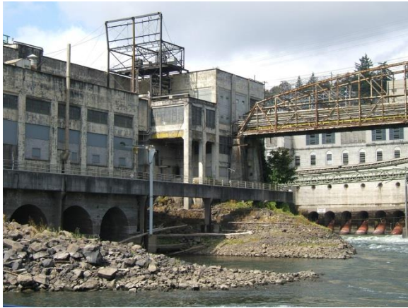
Mill A (left) and Sullivan Power Plant (right) (Photo courtesy of Sandy Carter)
